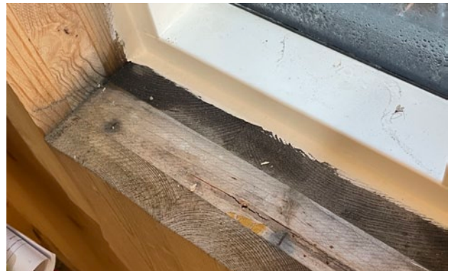
Figure 32. Unprotected window end grain
