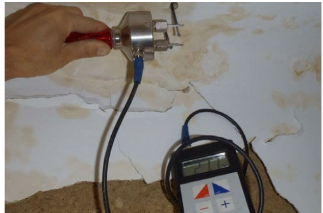
Figure 35. Measuring after water damage
