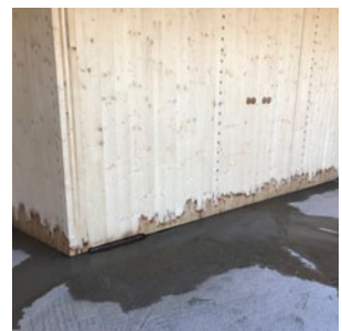
Figure 31. Exposed wall end grain on concrete foundation
